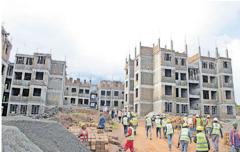
Workers at an affordable housing project site in Bahati, Nakuru County on May 22, 2024. JOHN NJORGE
